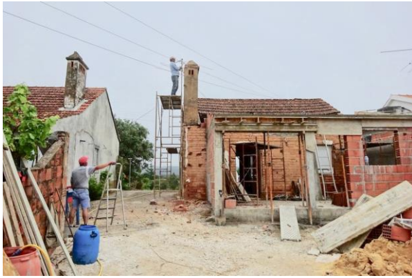
The chimney came down from the outside...
